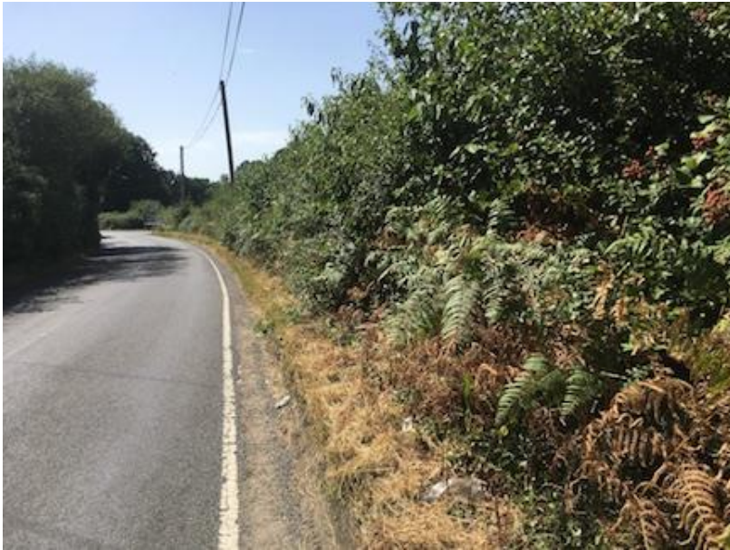
Plate 10: Failed Roadside Hedge
