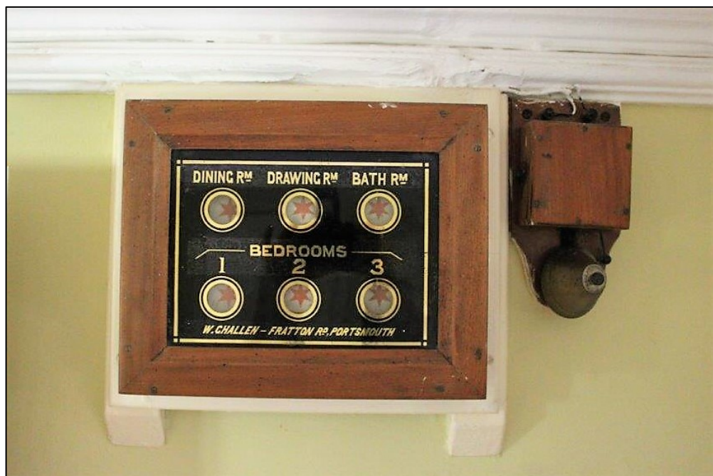
Photograph 23 Service call box in the older wing
