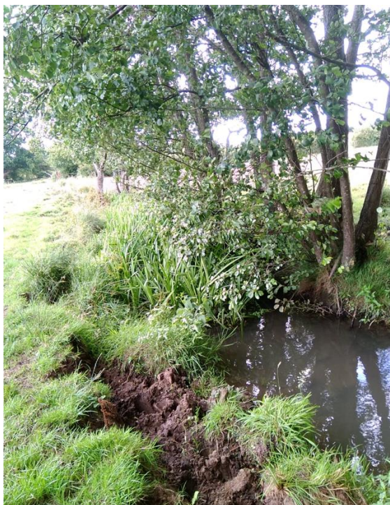
Plate 7: Reach 6. Southern channel poaching
