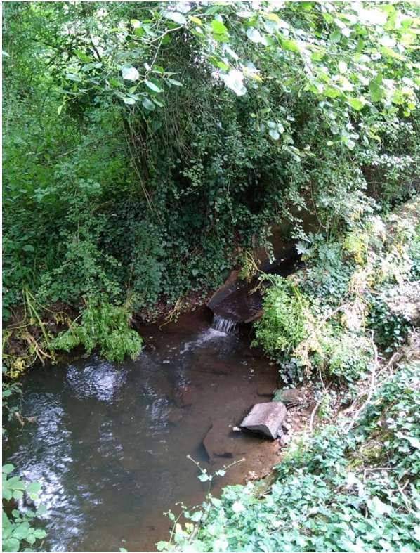
Plate 32: Reach 1. Confluence with Reach 3, barrier to fish migration and artificial (concrete half pipe) channel.
