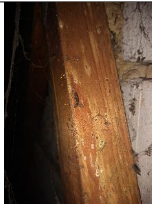
Photograph 8. Fresher dropping inside loft void
