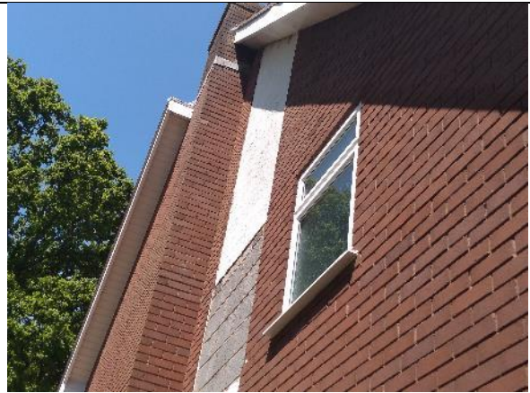
Photograph 6. Gaps were present to the flashing on the south-west elevation
