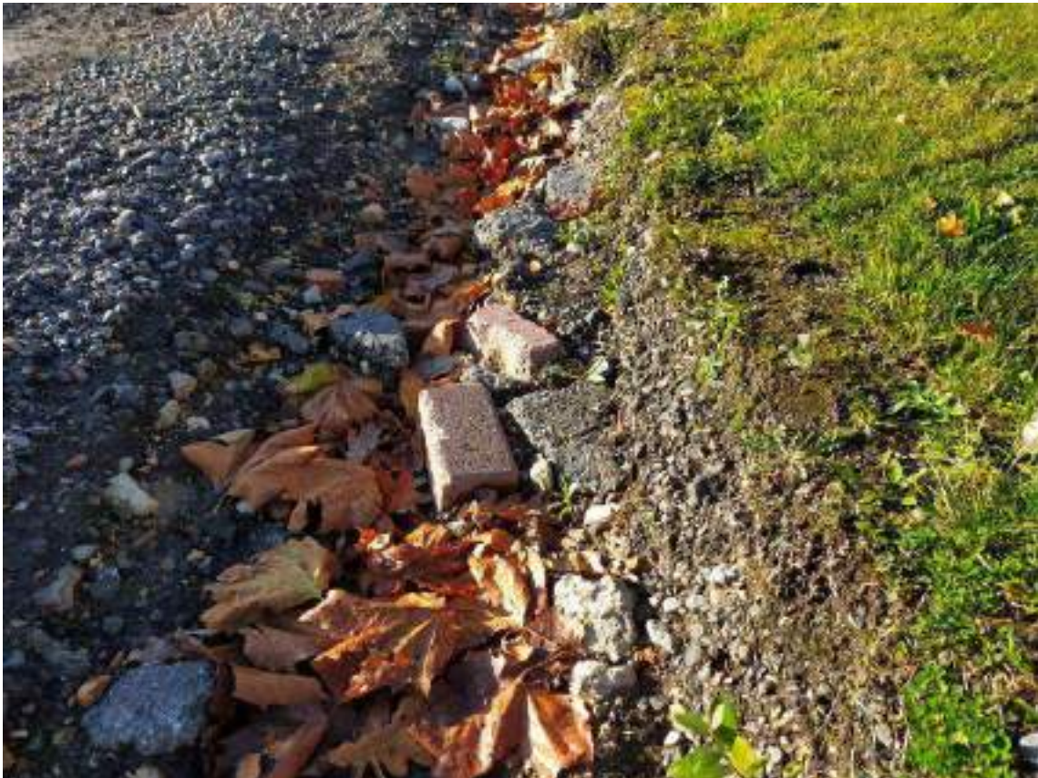
Photograph 28: Detailed view showing construction waste fill exposed beneath road plainings.
