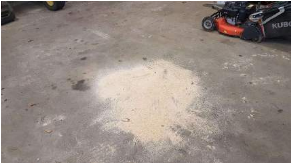
Photograph 7: General view ground floor workshop floor including sawdust covered recent spill.
