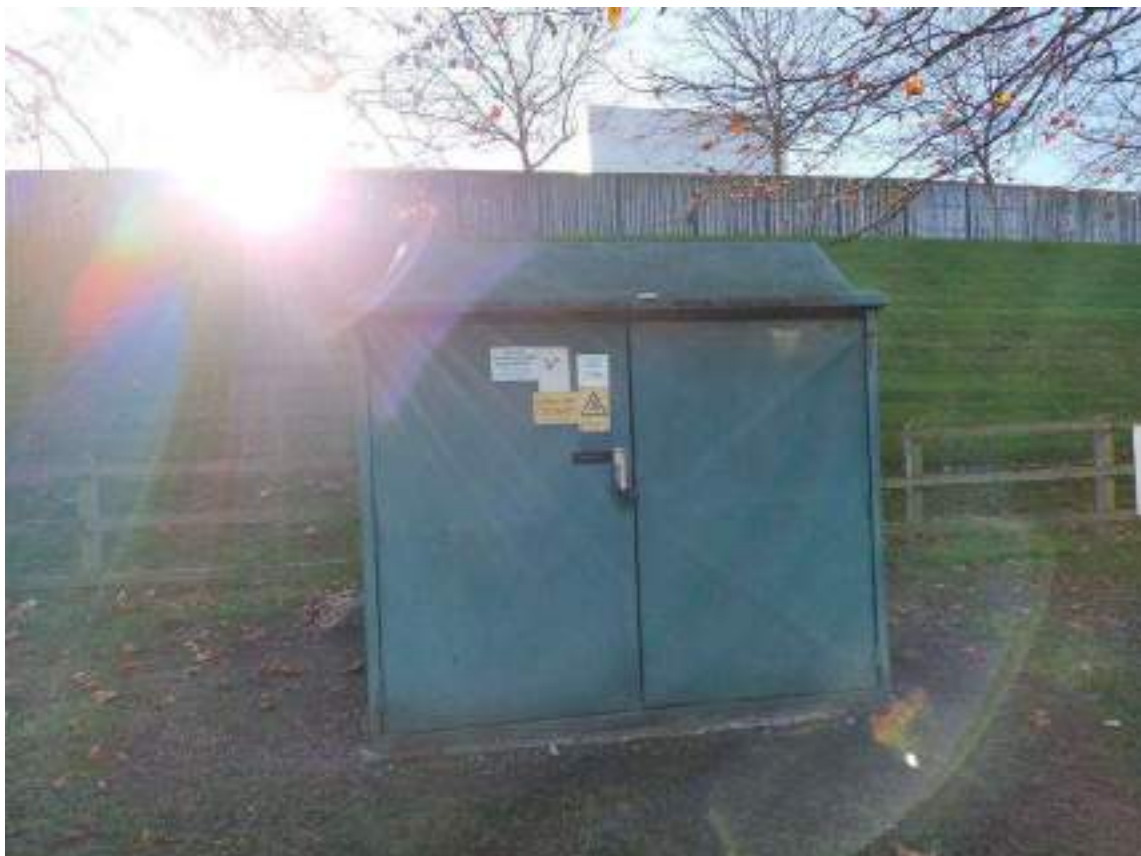
Photograph 26: General view South showing SSE plant off Marshall Drive.
