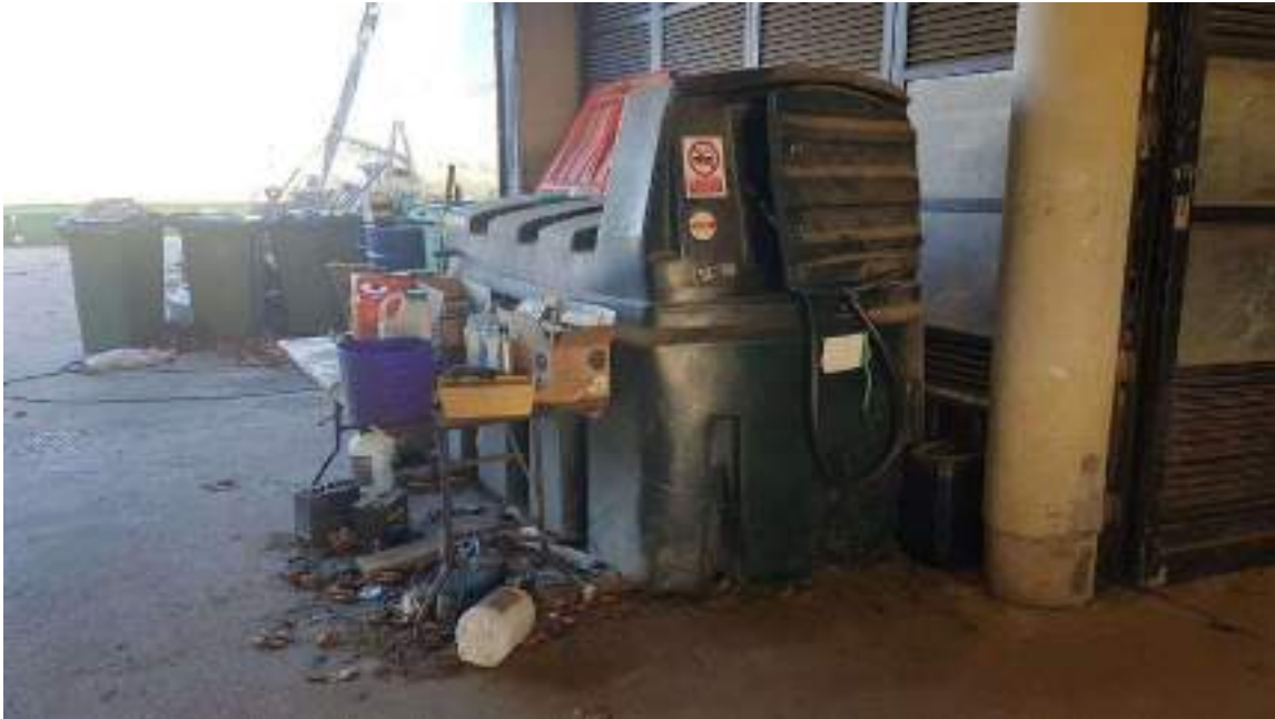
Photograph 9: General view ground floor access tunnel showing fuel storage tank.
