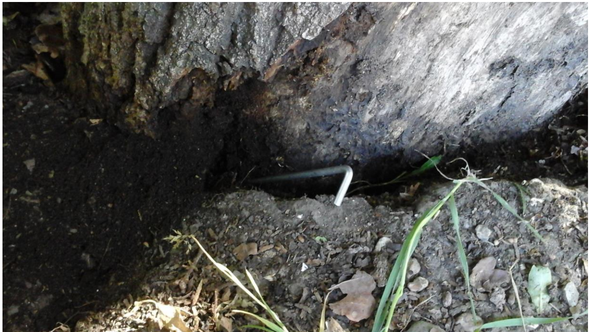
Degradation of exposed heartwood present on tension side and below the functional section.
