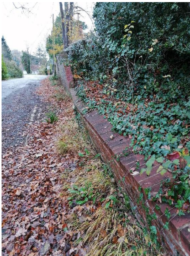
Photograph 2: Leaning wall adjacent to tree T1
