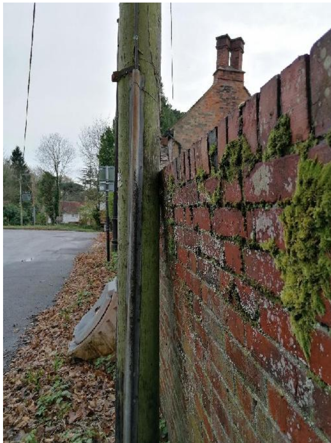
Photograph 6: Leaning wall and utility poll close to tree T2
