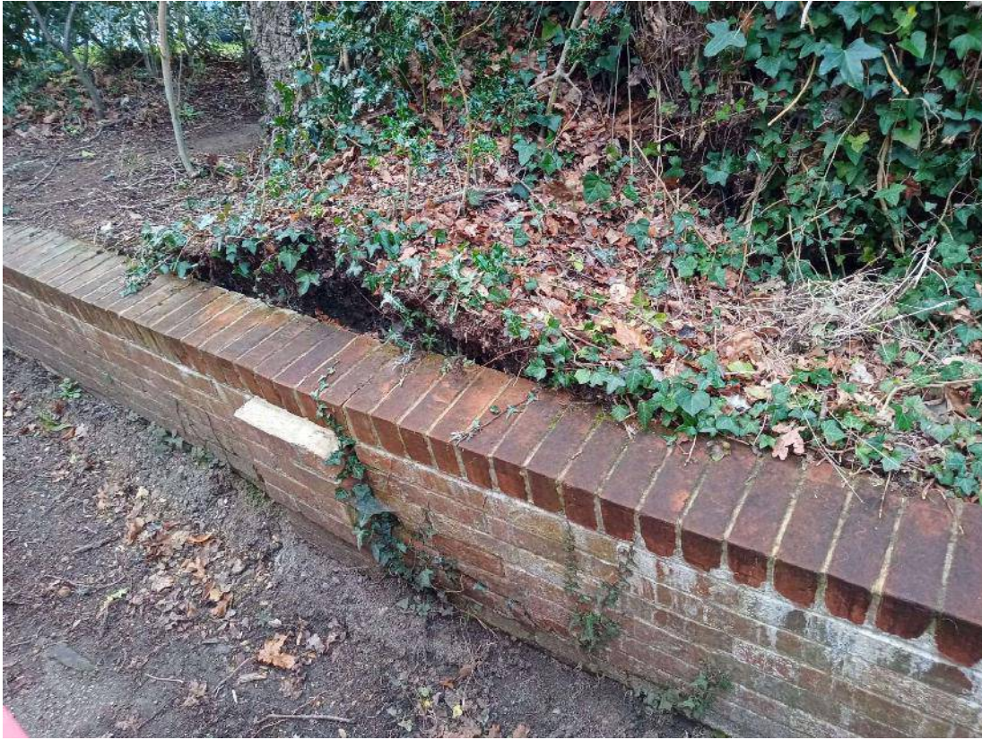
Photograph 5 – Proximity of mature tree behind wall in Length B
