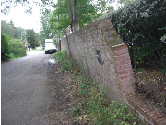
Severe leaning at the north end of the wall
