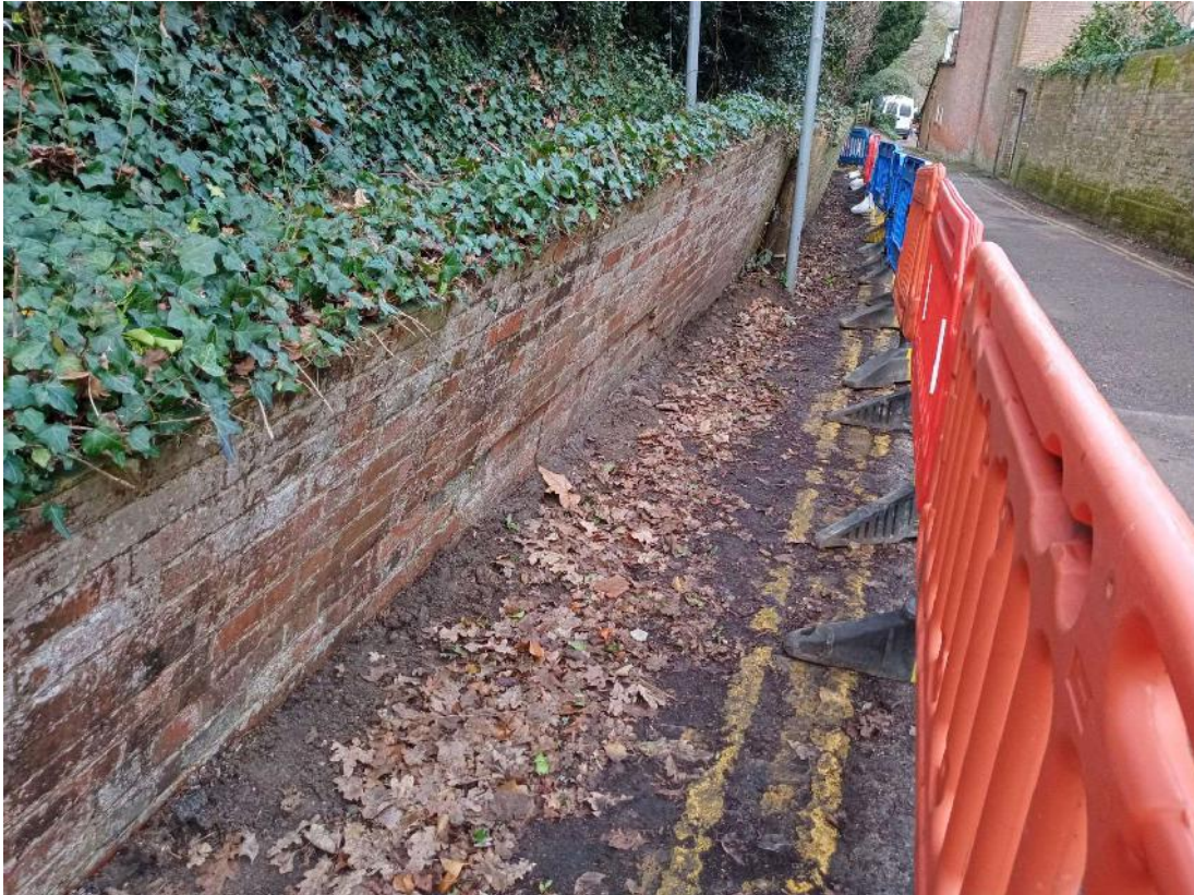
Photograph 6 – View along wall Length B showing shear failure along base of wall
