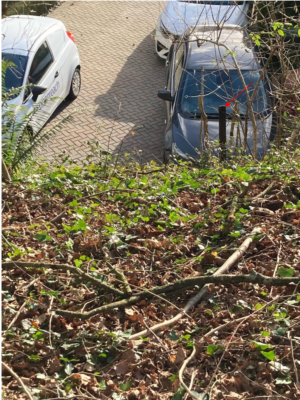
SAL4 Metal post identified by red arrow with car parking area below.
