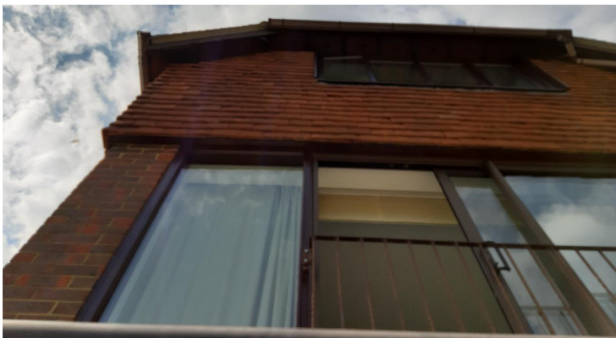
Photo 3: Gaps under hanging tiles to the south-east elevation
