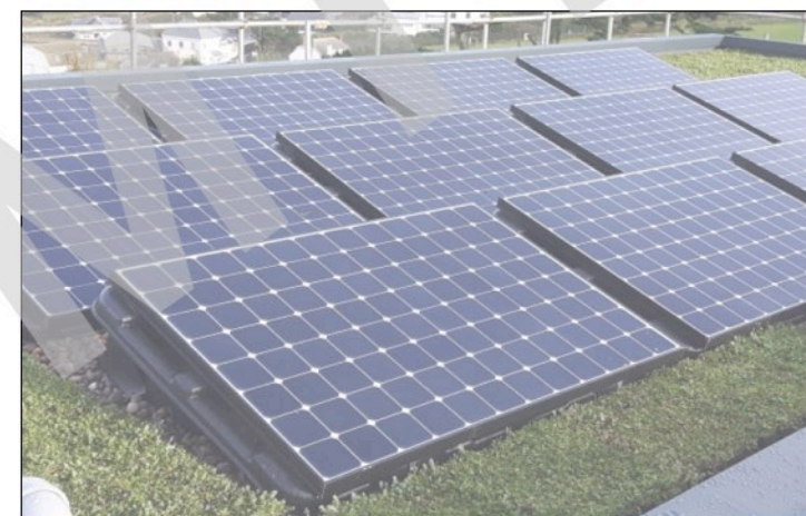
Solar PV Example
