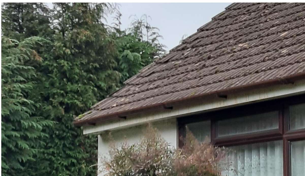
Photo 2: raised tiles on the roof 2020
