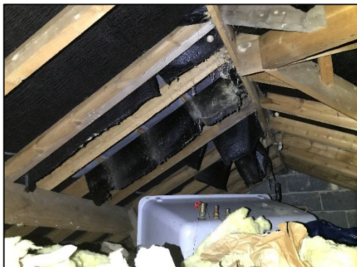
Figure 10: Internal void with damaged/missing bitumen felt lining
