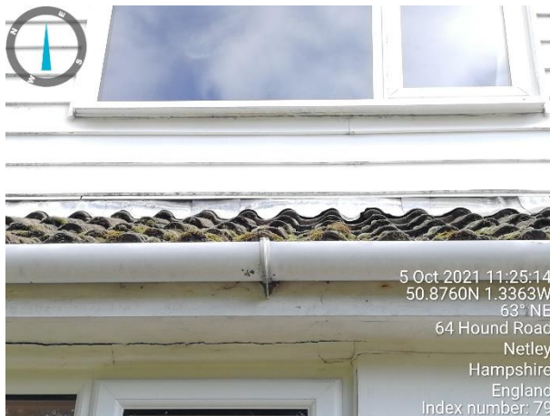
Photograph 31: View of some lifting in the lead flashing below the dormer on the rear of the property.
