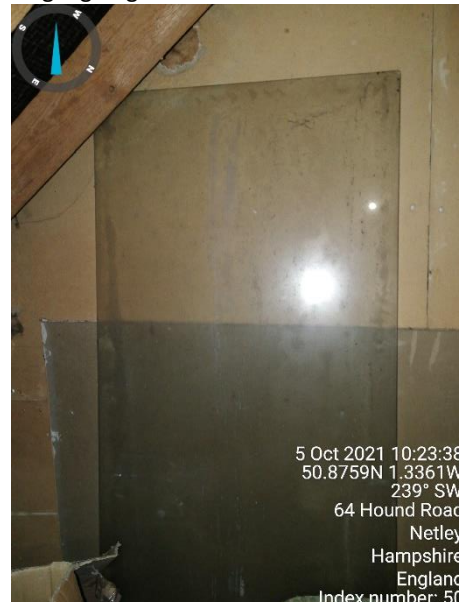
Photograph 6: Loft space within southern aspect of house and a pane of glass with urine staining present. Thought likely from rodents due to chewed MDF board above.
