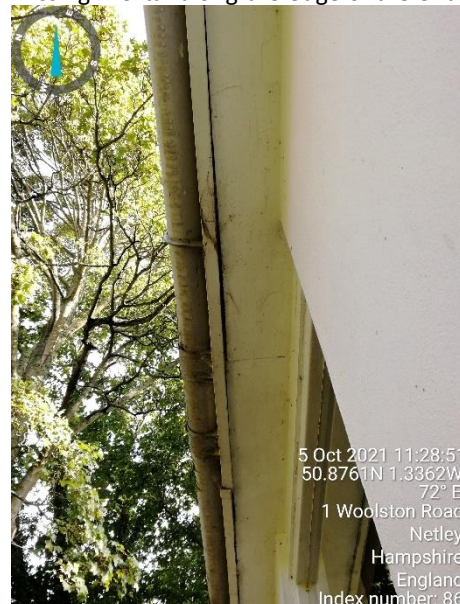
Photograph 36: View of the soffit along the northern elevation of the garage with gaps between the fascia and soffit board.
