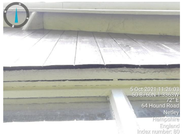
Photograph 32: View of a gap from missing render behind the shiplap located on the garages western gable end.
