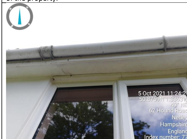
Photograph 29: View of PVC window to the rear with a crack above located just under the soffit.
