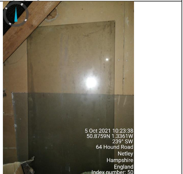
Photograph 6: Loft space within southern aspect of house and a pane of glass with urine staining present. Thought likely from rodents due to chewed MDF board above.
