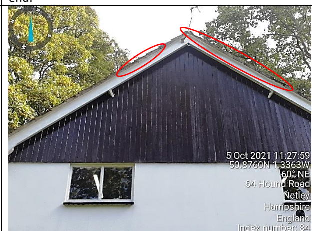
Photograph 34: View of garages western gable end and missing mortar along the edge of the end tiles.
