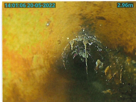
Fig 1.2: This shows the root ingress within the SVP pipework.
