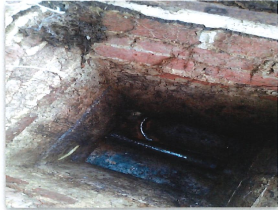
Fig 2.2: This shows the root ingress located within the manhole at the front of the customers property.
