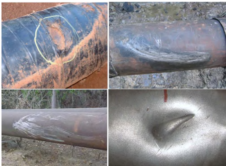
Figure 24. Examples of Severe Damage to Pipelines
