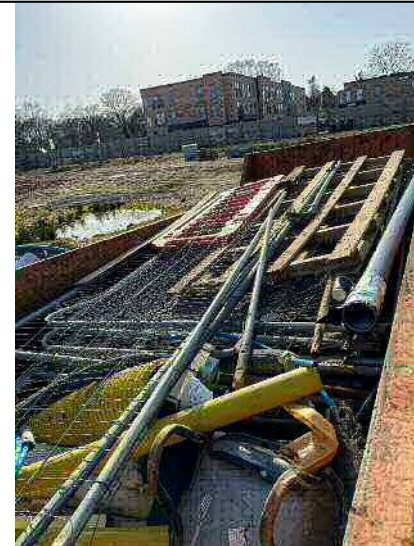
Photograph 8 – A view of the waste skip located centrally on site.
