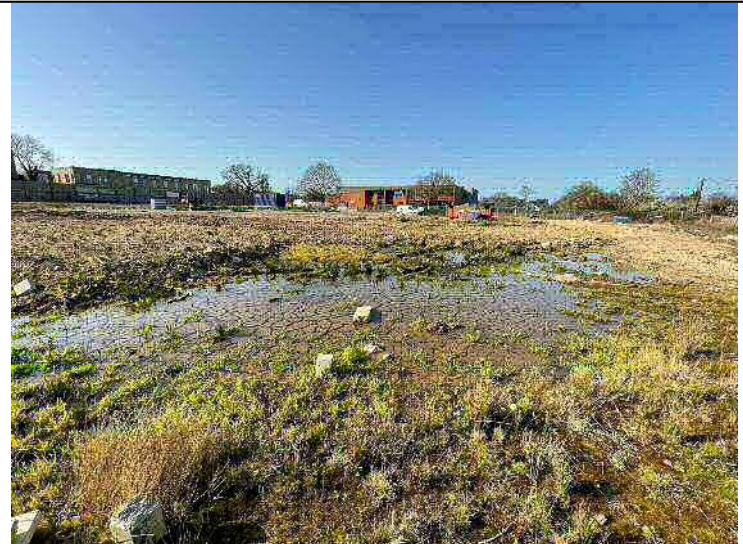
Photograph 4 – A view of the ponding in the south of the site.
