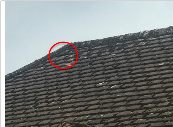
Gaps under tiles near ridge
