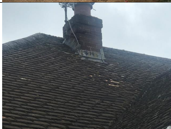
Chimney with lifted lead flashing
