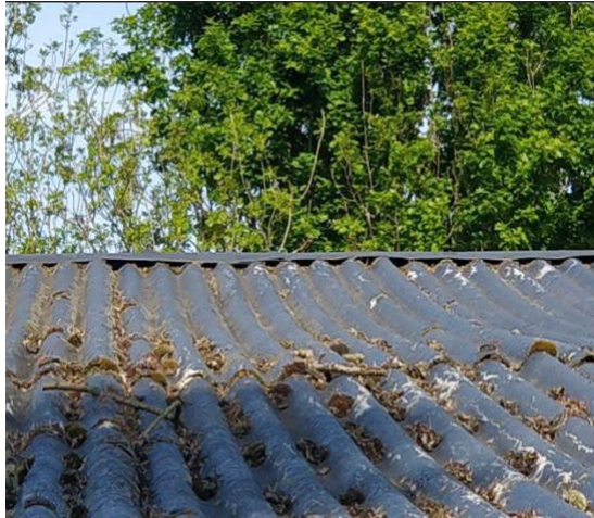
Figure 9. View of gaps underneath metal ridge.
