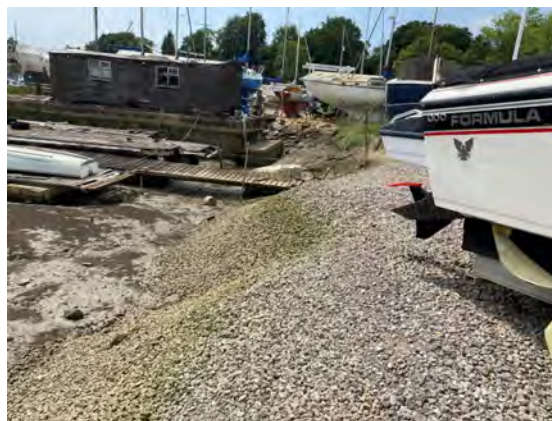
Photo 10: Southern boundary with no sheet pile wall or gabions
