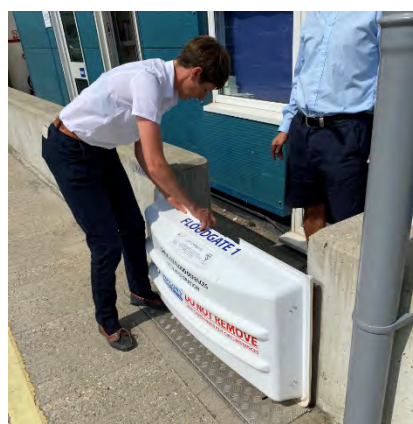
Photo 12: Example of floodgate protecting The Workshops
