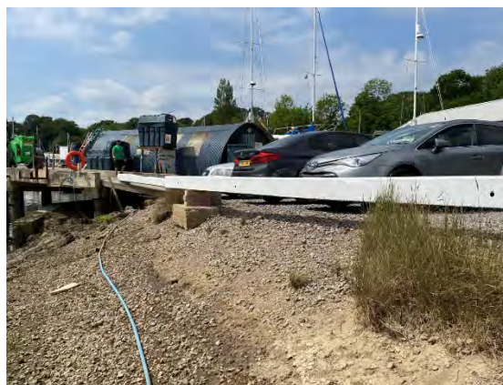
Photo 8: No sheet pile wall or gabions in the centre of the site. During high tides water ingresses onto the site from this area.
