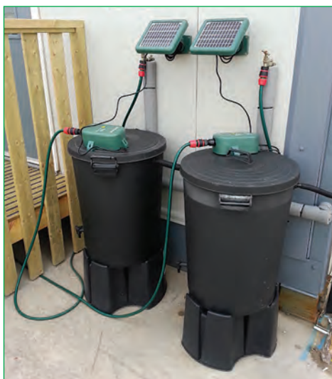
Figure 4.51 Greywater capture with solar powered pumps (courtesy BAM Nuttall)
