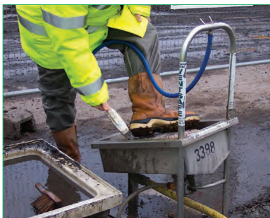
Figure 4.60 On-site boot wash facility (courtesy Galliford Try plc)
