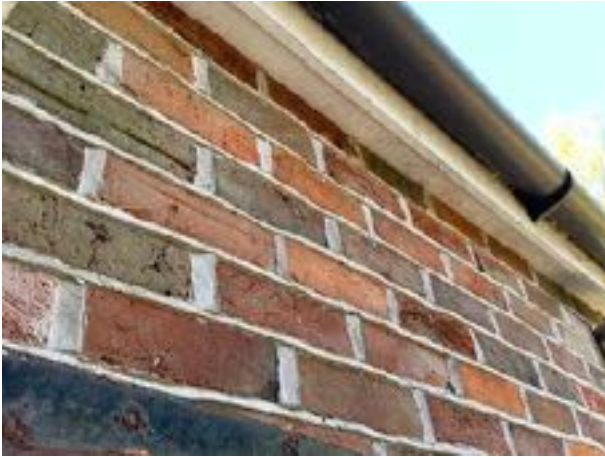
Figure 13 - No gaps between soffit and wall
