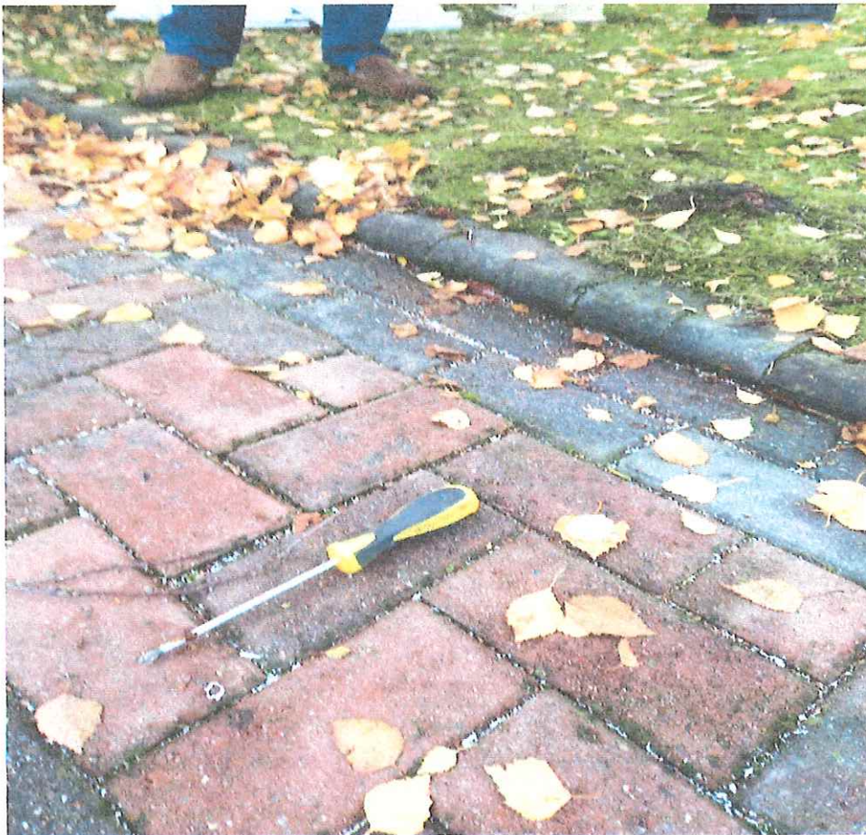
Drive blocks and kerbs lifting from roots
