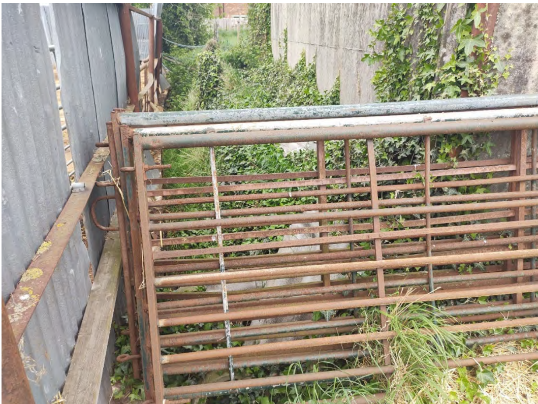
Plate 16 – Broken asbestos cement adjacent to western elevation of the northernmost barn
