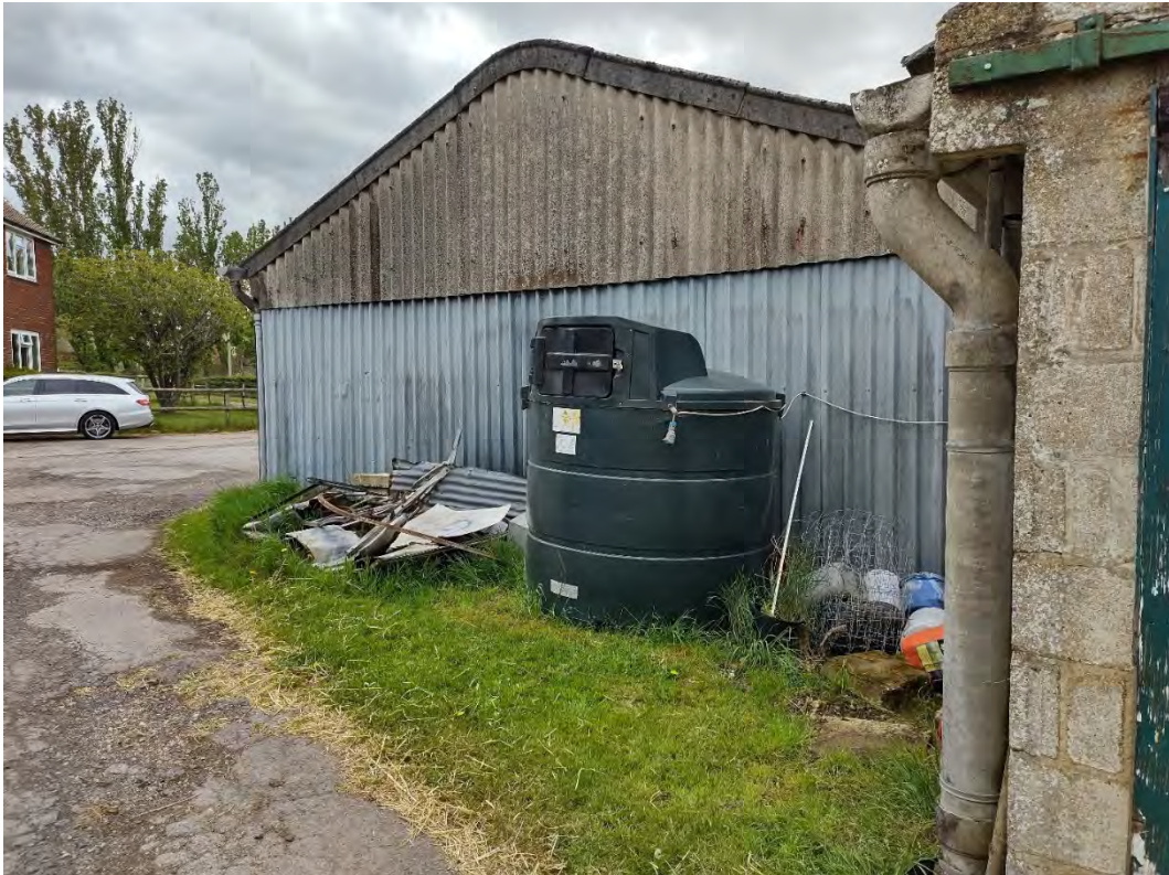
Plate 11 – Diesel AST and location of former steel diesel AST
