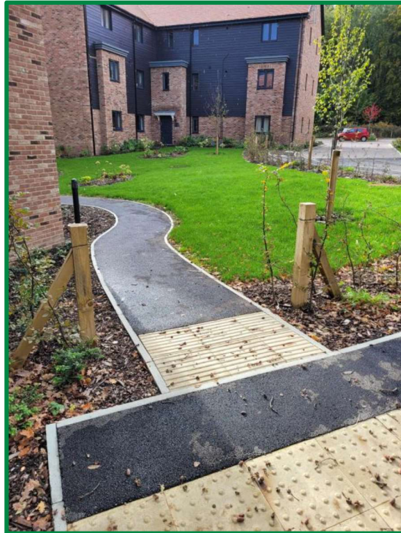
Photo 13 – Bollards Substituted for Fence Posts
