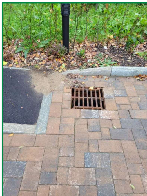
Photo 16 – Evidence of Sediment Accumulation
