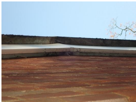
Dead-ended gap behind bargeboards on side gables
