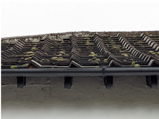
Picture 5: Missing mortar at front of end tile.
