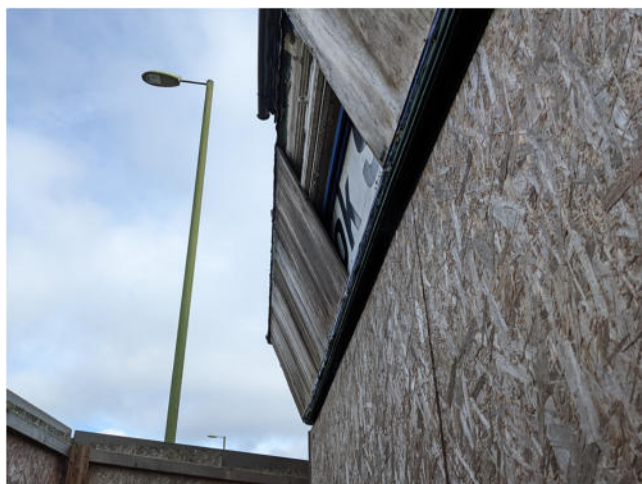
Picture 4: Broken boarding Building B1 western aspect.
