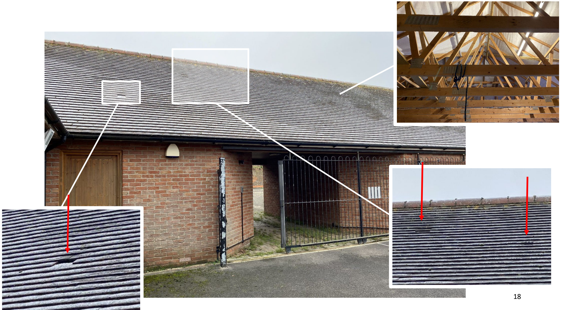
Figure 5. View of the eastern (rear) elevation with annotations of internal areas and any PRFs recorded (taken December 2022).
