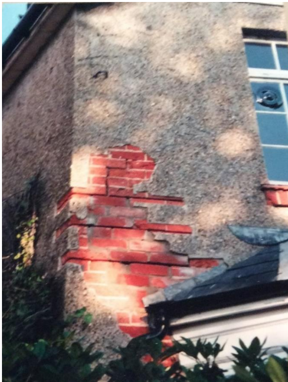
Figure 7: Subsidence on the corner of the front/west corner (footing to plate) sufficiently severe to lift the render. (Category 4/5, BRE Digest 251 classification).
