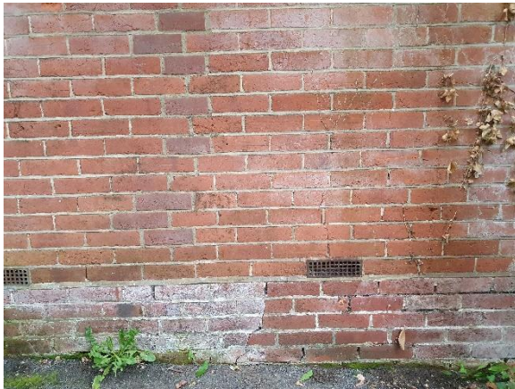
Figure 5: The ground floor extension (entrance and hall) on the north elevation is located on the diagonal fault line (subsidence) from the south elevation of 13 Satchell Lane (visible cracking) to the north elevation of 15 Satchell Lane. The footing of the loadbearing dividing wall (south/north elevations) at 15 Satchell Lane is located on the diagonal fault line and has been the subject of two interventions for subsidence since 2002.
