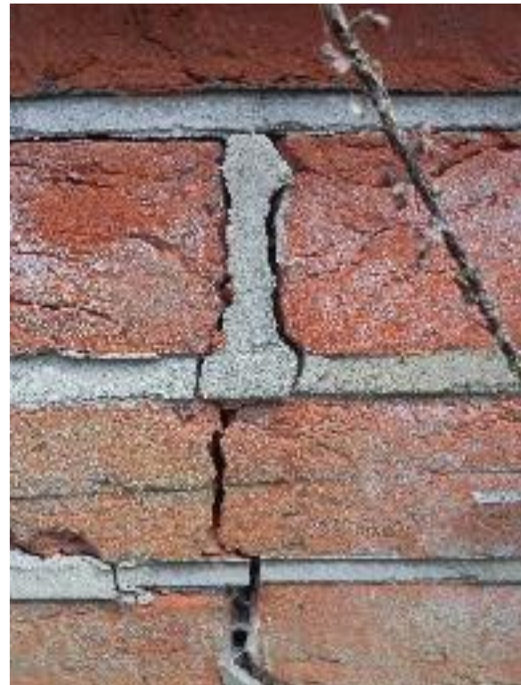
Figure 8: Visible signs of subsidence below the bay window (above) to the footing and horizontally to the corner of the west/front elevation.
