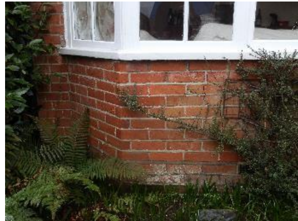
Figure 6: Subsidence on the corner of the front (south/east corner) travels from the dampproof course to plate level. The south and east elevations of 15 Satchell Lane are the areas most affected by subsidence (Category 4/5, BRE Digest 251 classification). Visible signs of subsidence from just below the bay window (above) to the footing.
