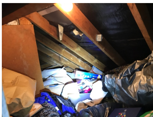
Figure 7 – tears in bitumen lining and hanging folds
