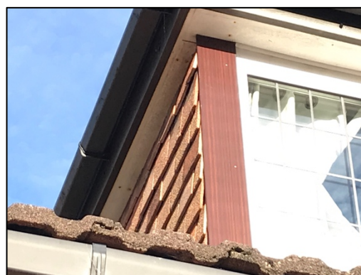
Figure 6 – gaps under hanging tile on dormer windows
