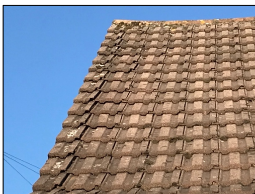
Figure 5 – lifted interlocking concrete tiles
