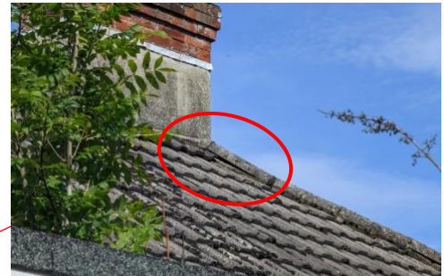
Gap underneath the ridge tiles on the eastern elevation
