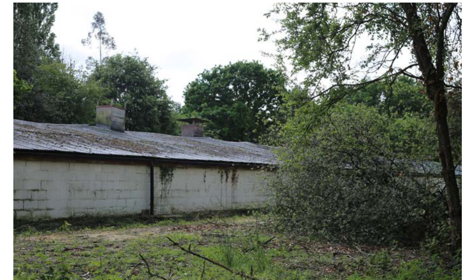
The site is in poor condition
