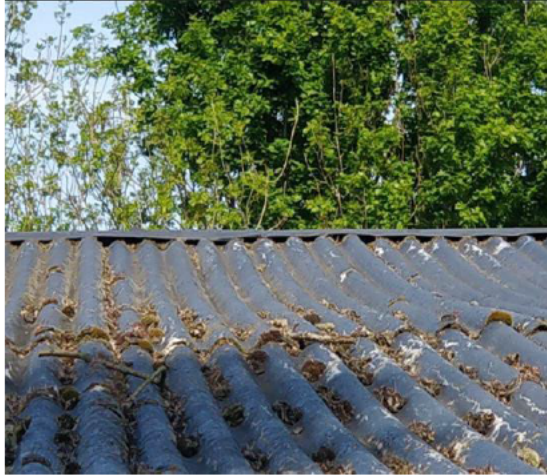
Figure 9. View of gaps underneath metal ridge.
