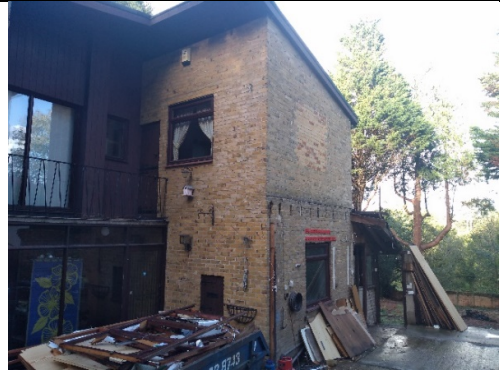
Photograph 4. Gaps in the brick work on southeast elevation of B1
