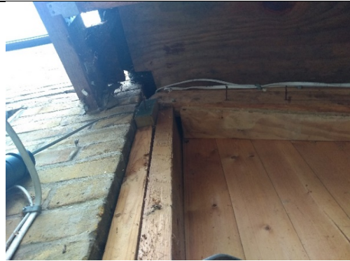
Photograph 2. Gaps in the wooden porch on southeast elevation of B1
