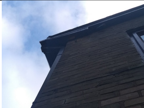
Photograph 3. Wooden soffit box with gap northwest corner of B1
