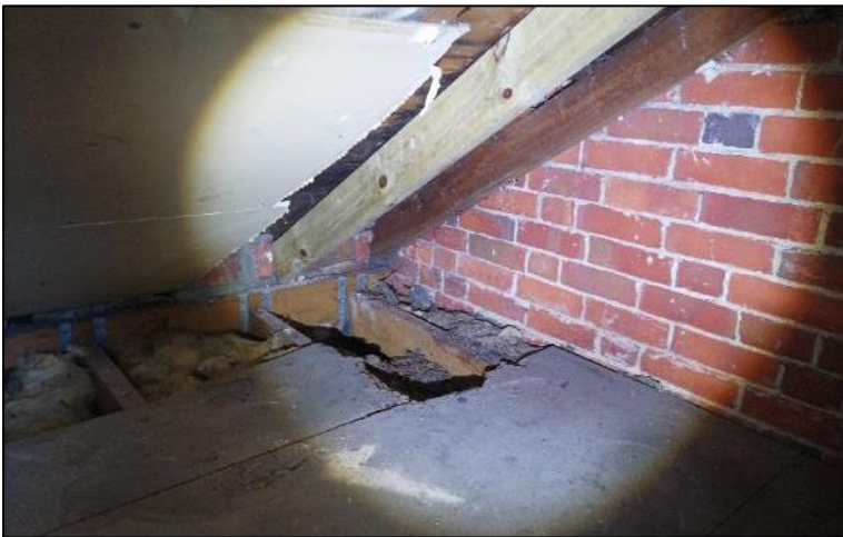
Figure 7 – eaves on southwest elevation with deteriorating timbers
