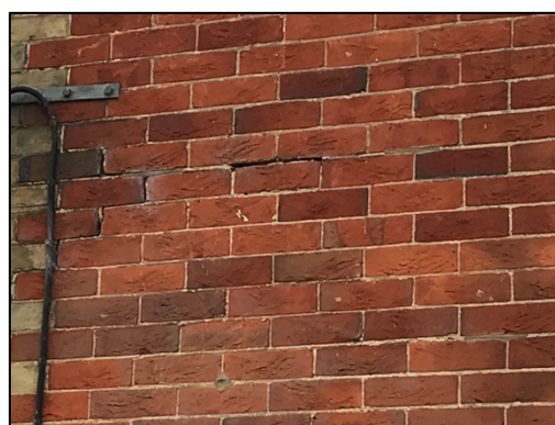
Figure 10 – gap present in the brickwork
