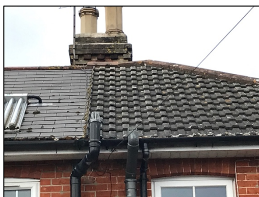
Figure 9 – lifted roof tile with gap underneath
