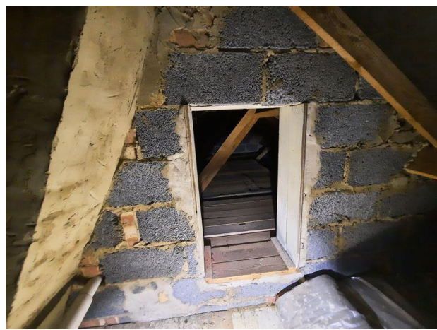
Plate 4.10: Additional Loft Space Access
