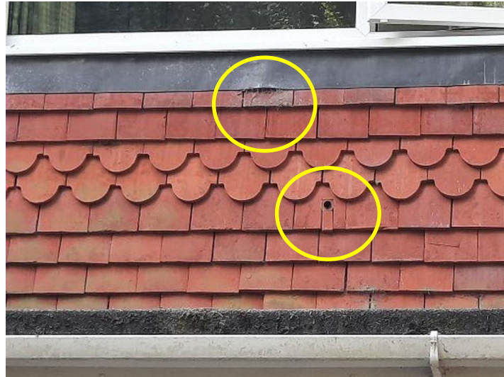
Plate 4.3: Gaps and Holes within the Hanging Tiles (Northern Elevation).
