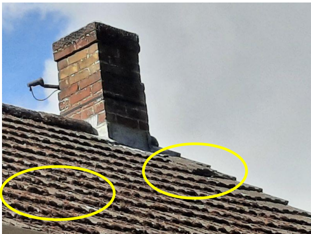
Plate 4.4: Gap under Lifted Tile
