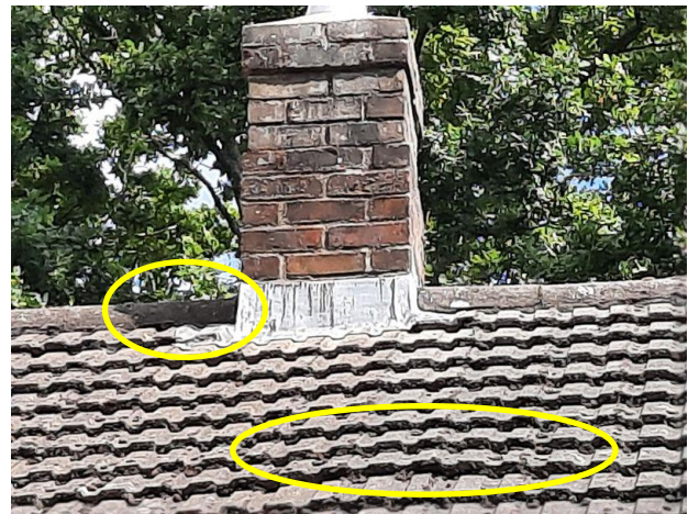
Plate 4.5: Warped Tiles and Gap under Lead Flashing
