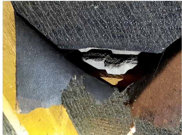
Plate 4.13: Torn Felt with Access to Roof Tiles
