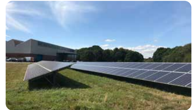
Solar farm, building 9 in background
