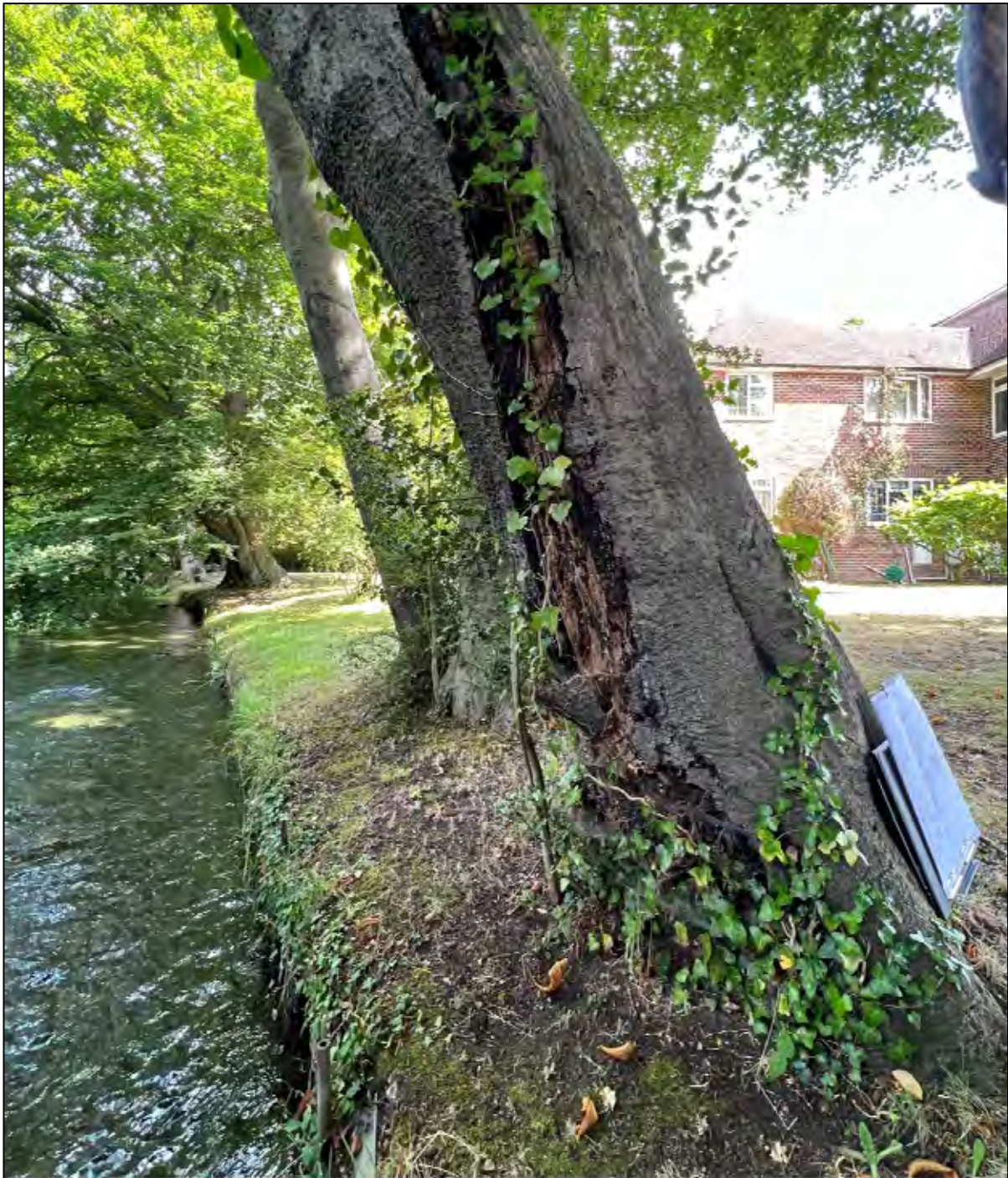
Figure 3: An example of other severe defects in the trees within this broad group, that prevents them being retained without significant management works.
