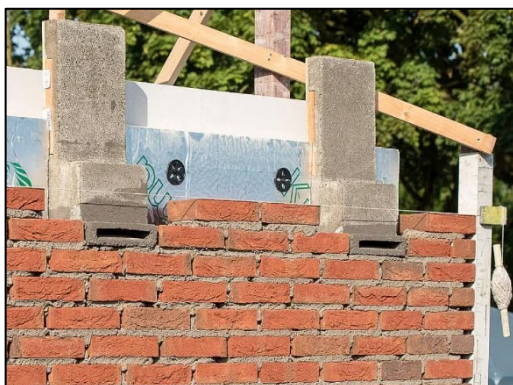
Figure 17: Example of Build-In Woodstone Bat Boxes integrated into fabric of wall
