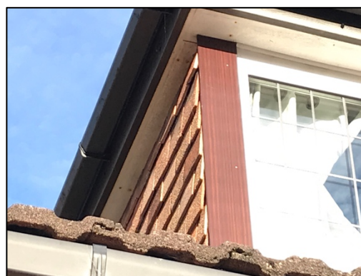
Figure 6 – gaps under hanging tile on dormer windows
