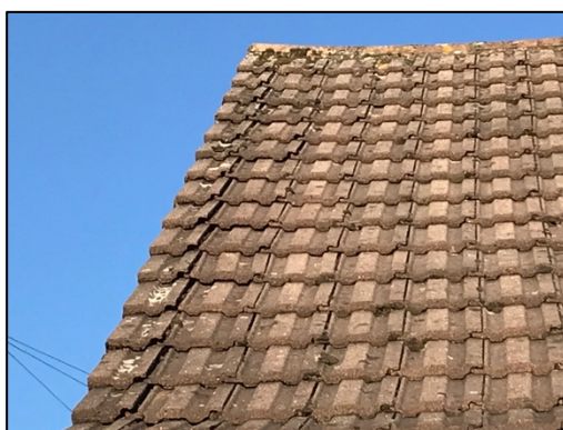
Figure 5 – lifted interlocking concrete tiles
