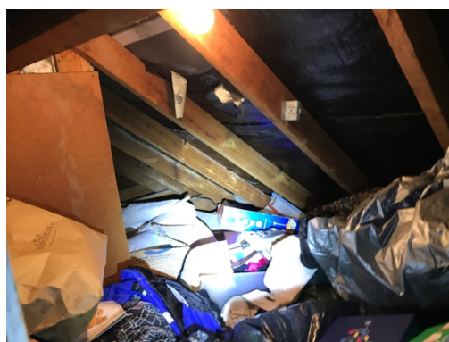
Figure 7 – tears in bitumen lining and hanging folds
