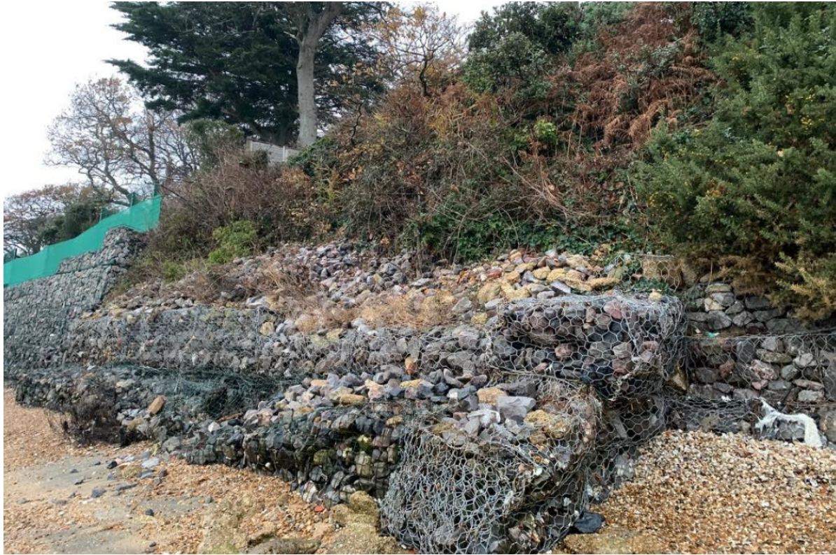
Further degradation of sea defence gabion wall (Feb 2022)
