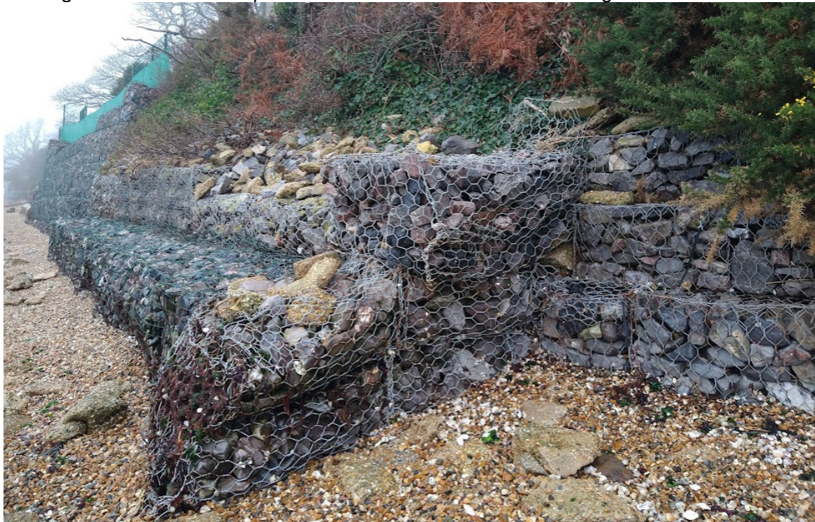
Poor condition of sea defence gabion wall (Sept 2022)
