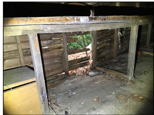
Figure 13 – holes in shed woodwork
