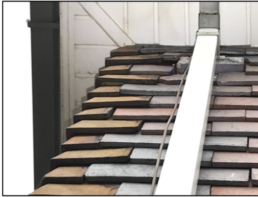
Figure 10 – gaps under hanging tiles on top half of elevations
