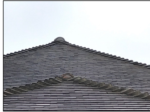
Figure 11 – lifted tiles on roof face of the main dwelling and south-eastern extension
