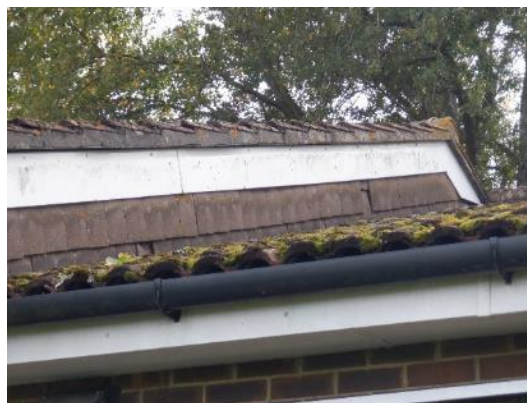
20. Uneven hanging tiles on the western gable (B2).
