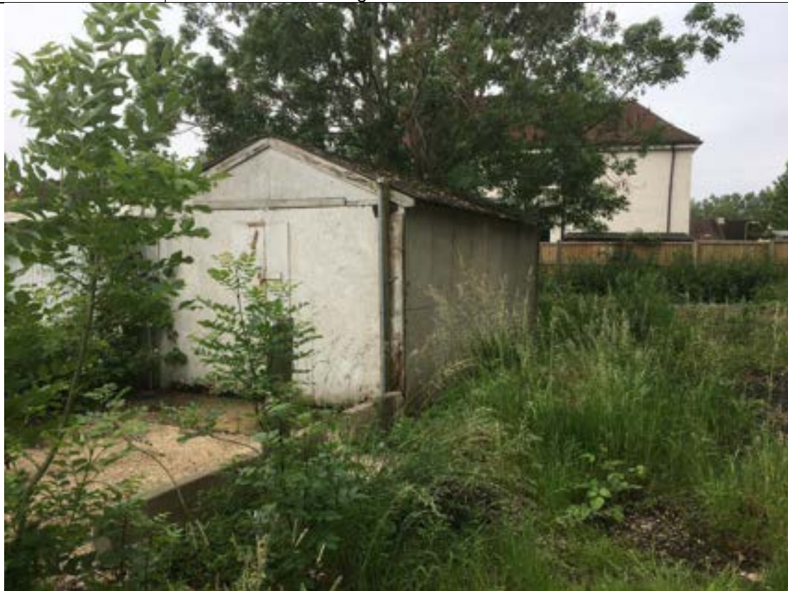
Photo 2: View Southwest of Garage with possible Asbestos Roofing materials
