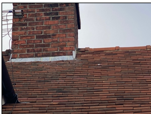
Figure 5 – gaps under roof tiles and under lead flashing
