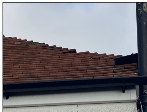
Figure 6 – missing mortar under hip tiles
