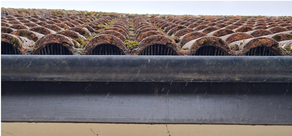
Picture 4: Showing the vent guards under the tiles
