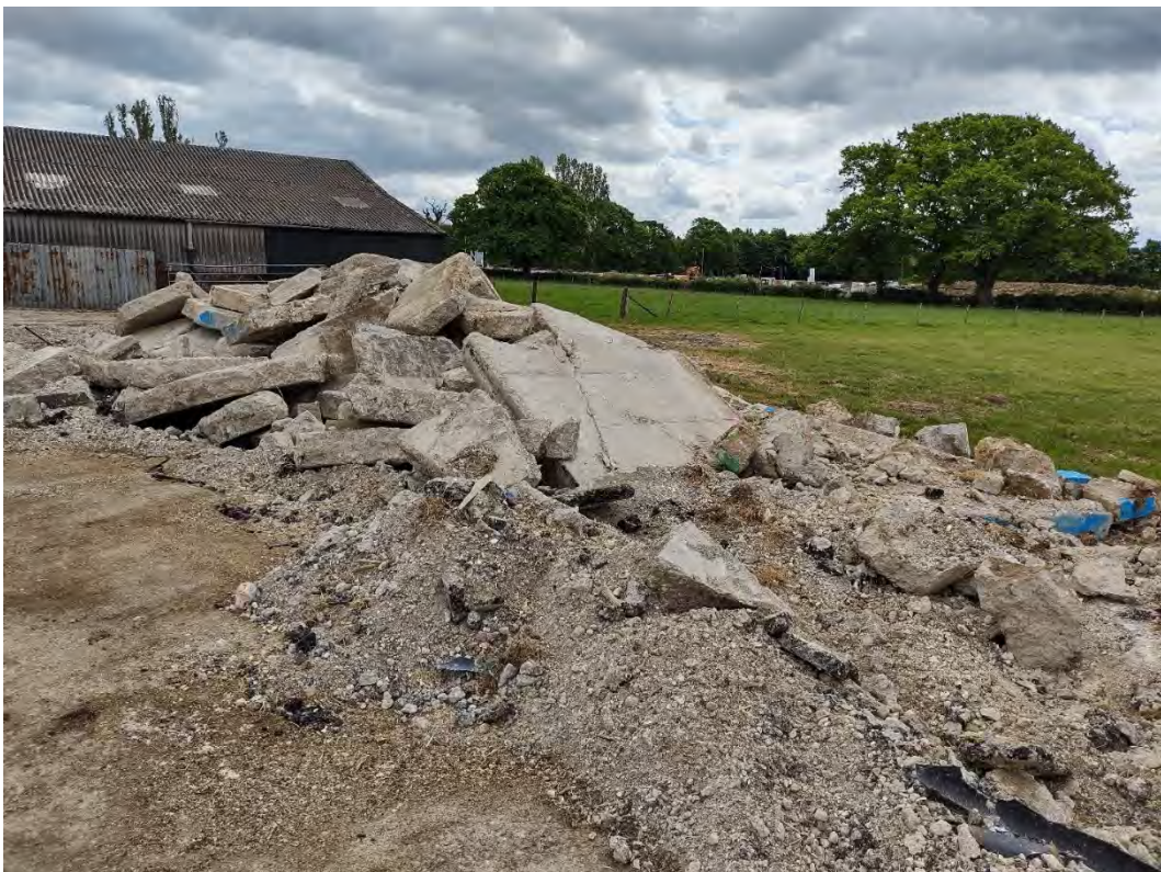
Plate 6 – Broken concrete from the former barn floor slab
