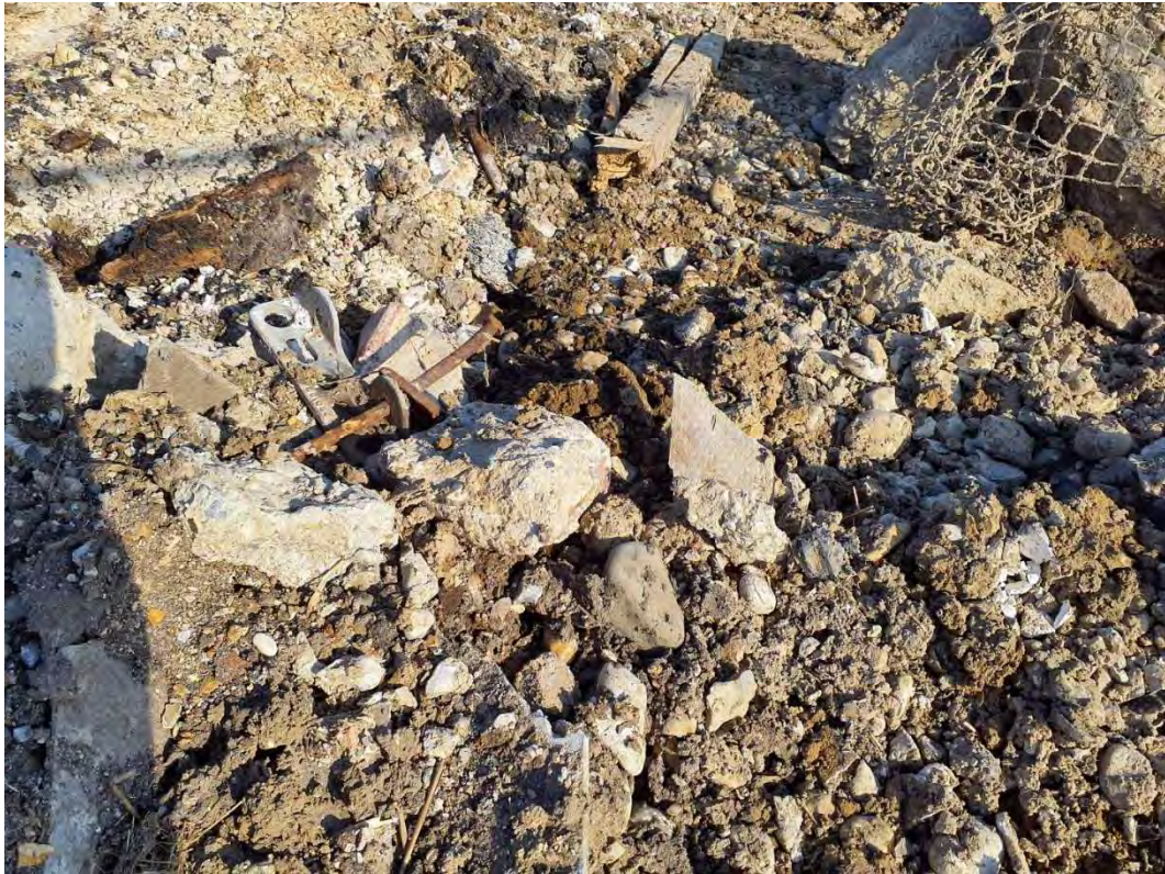
Plate 9 – Potential asbestos cement fragments north of TP109 on site surface
