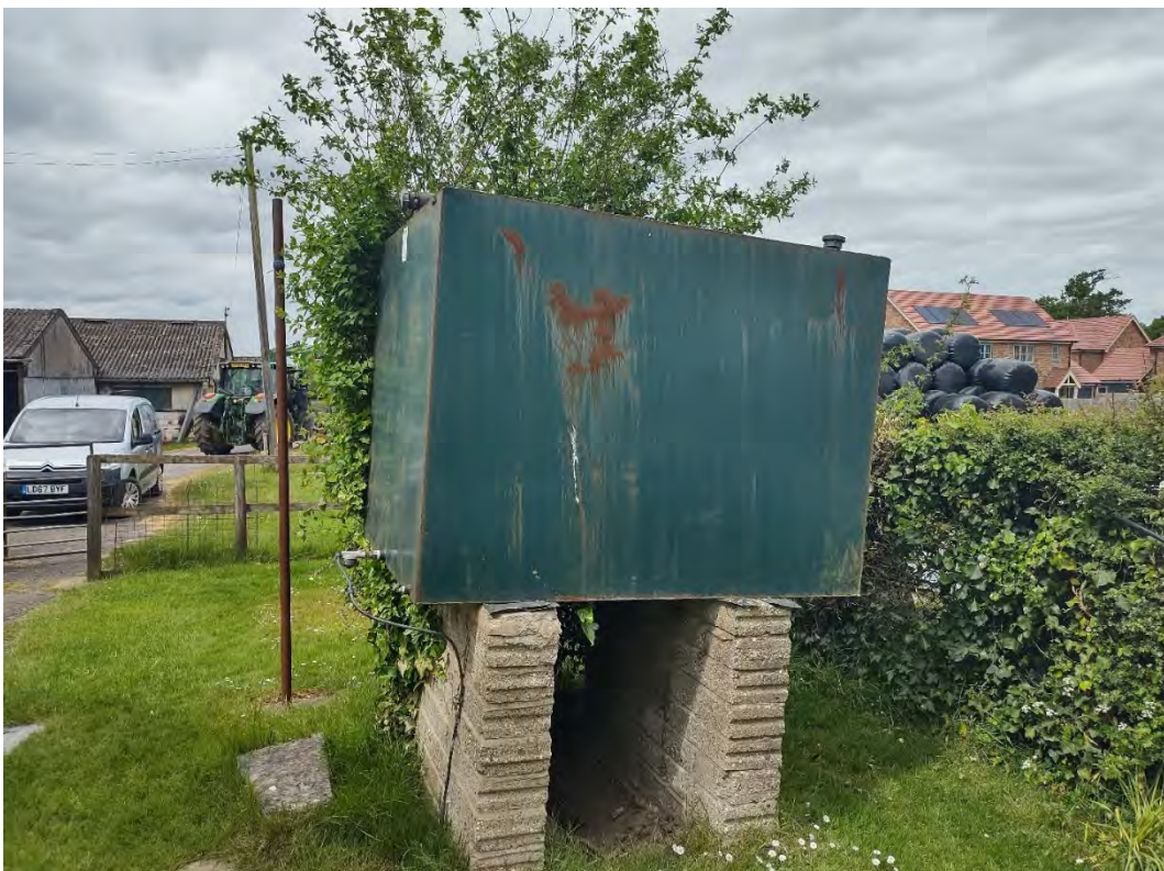
Plate 10 – Heating oil AST
